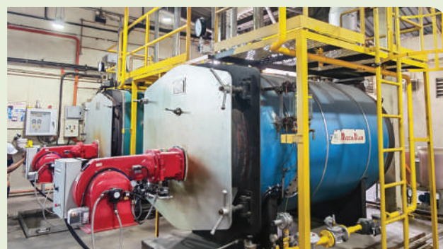
The upgraded dual-fuel boiler at the Pulau Indah facility
