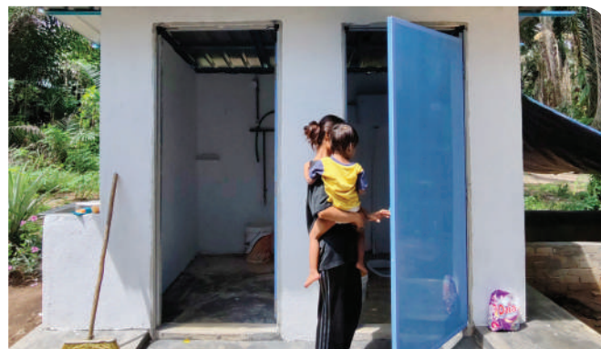
PPB sponsors building materials for the Orang Asli communities to build their own sanitation facility
