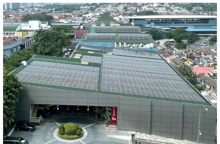
The installation of solar panels at Cheras LeisureMall contributes to the adoption of renewable energy and the reduction of carbon footprint
