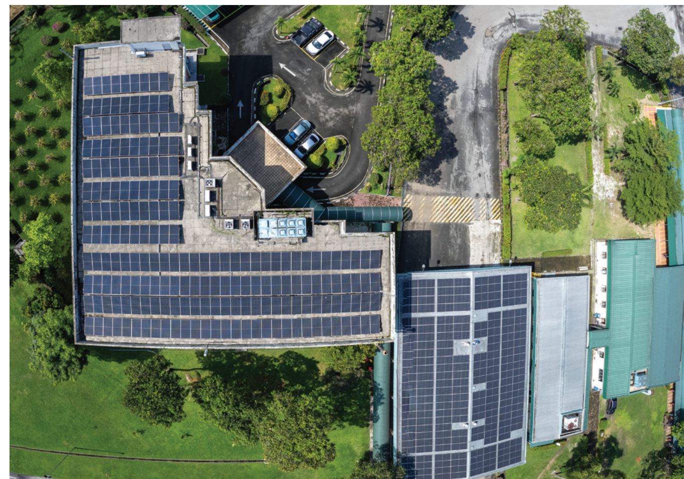
One of FFM's solar PV system commissioned in 2023
